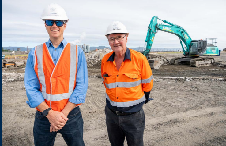
Construction of the Port Kembla Bulk Ethanol Terminal is overseen by Project Manager David Johnston and Construction Supervisor Gordon Rewell // PHOTO: PETER IZZARD
