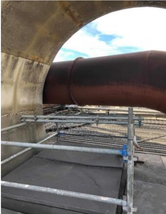
EPA ID 9 – No. 2 Gluten Dryer Baghouse
