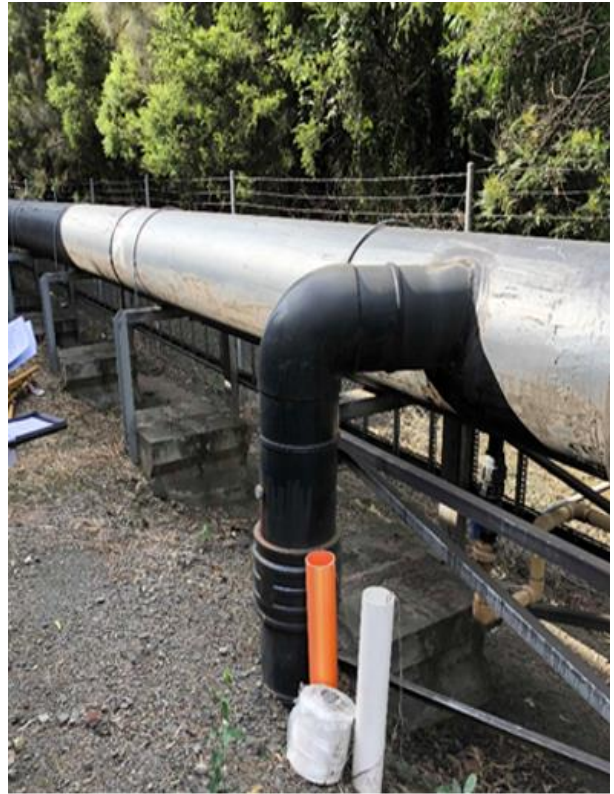
EPA ID 39A - Biofilter Inlet
