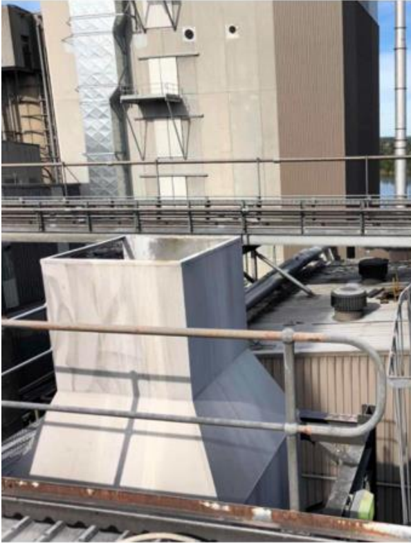
EPA ID 13 – No. 3 Starch Dryer Scrubber
