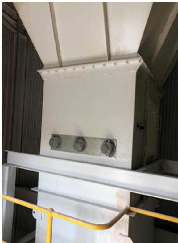
EPA ID 11 – No. 4 Gluten Dryer Baghouse
