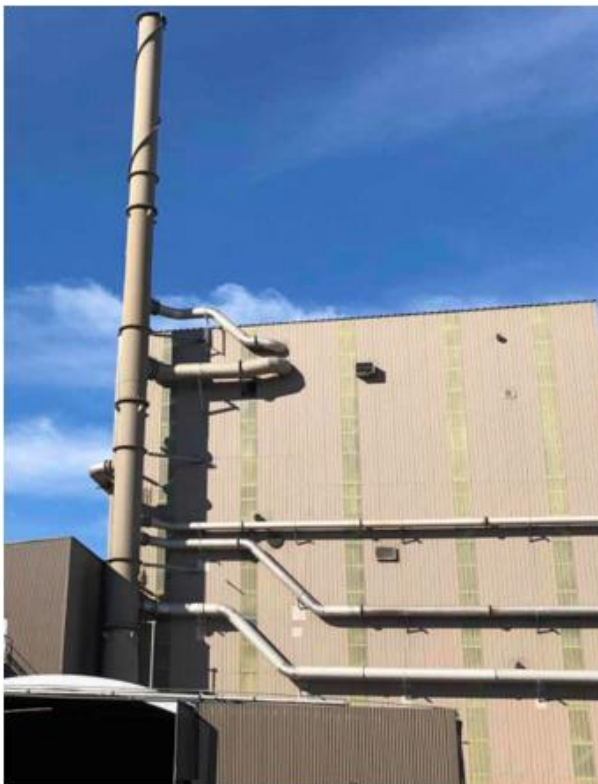
EPA ID 46 - DDG Pellet Plant Stack
