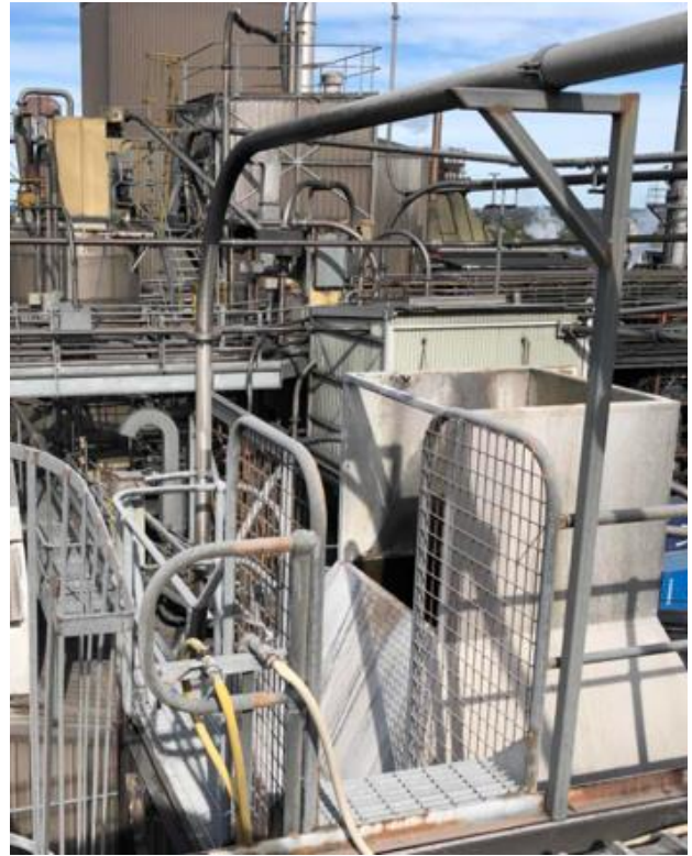
EPA ID 14 – No. 4 Starch Dryer Scrubber
