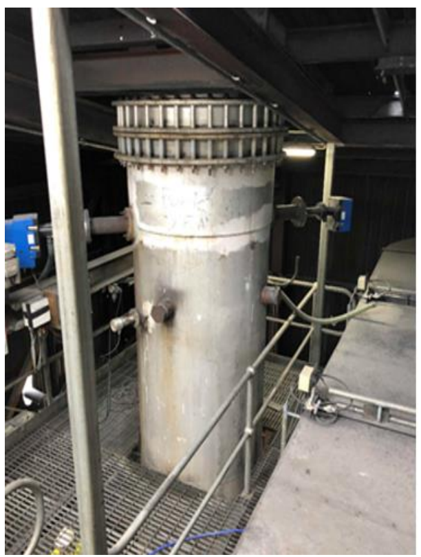
EPA ID 42 - Boiler 4
