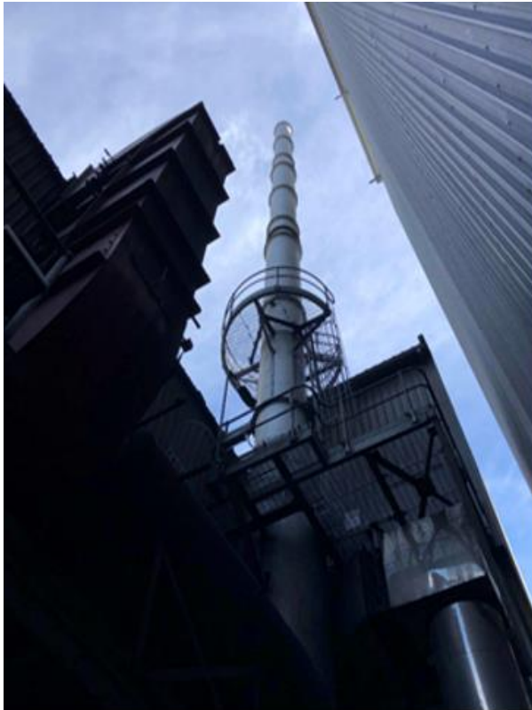
EPA ID 45 - Boiler 2
