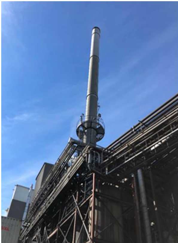
EPA ID 35 - Combined Boiler 5 & 6 Stack
