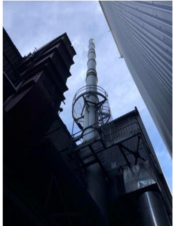
EPA ID 45 - Boiler 2
