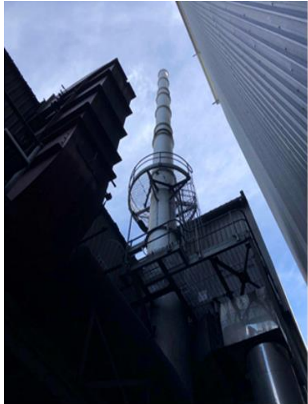
EPA ID 45 - Boiler 2
