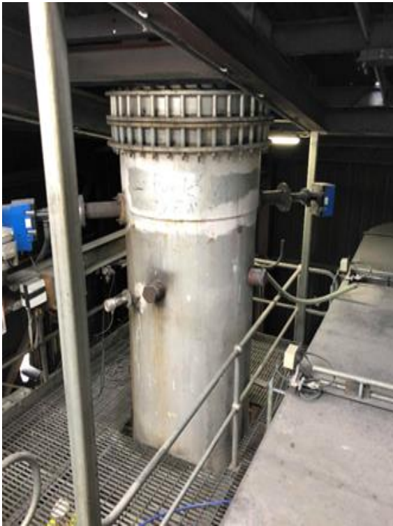
EPA ID 42 - Boiler 4
