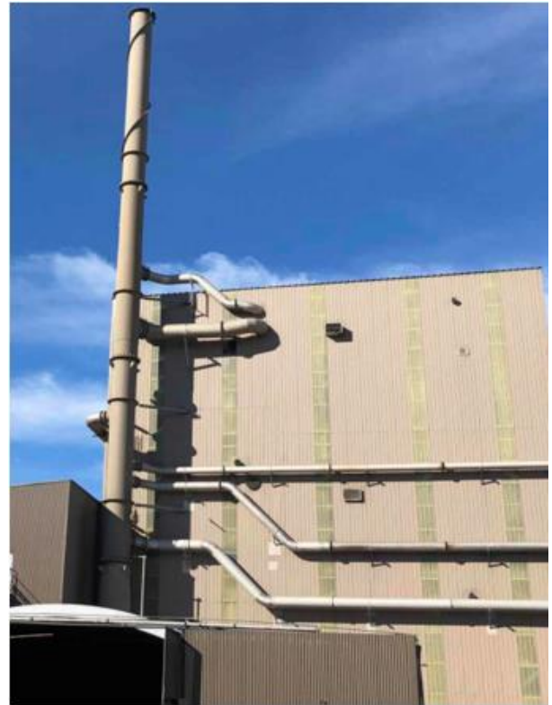
EPA ID 46 – DDG Pellet Plant Stack
