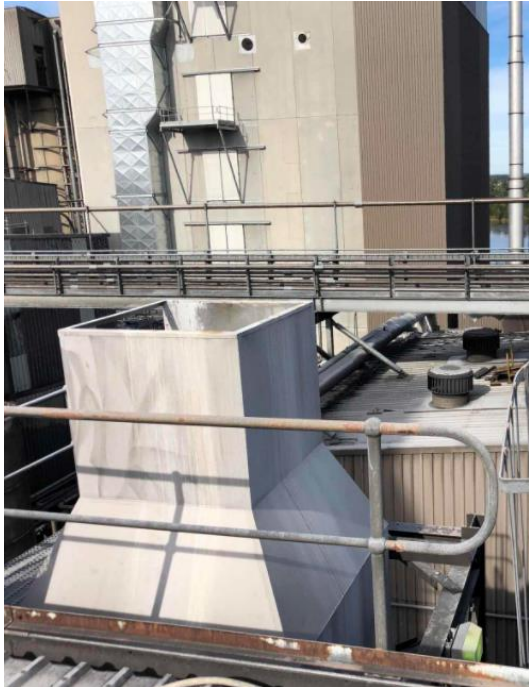
EPA ID 13 – No. 3 Starch Dryer Scrubber
