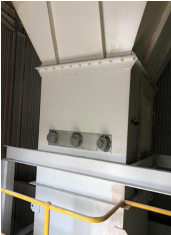
EPA ID 11 – No. 4 Gluten Dryer Baghouse
