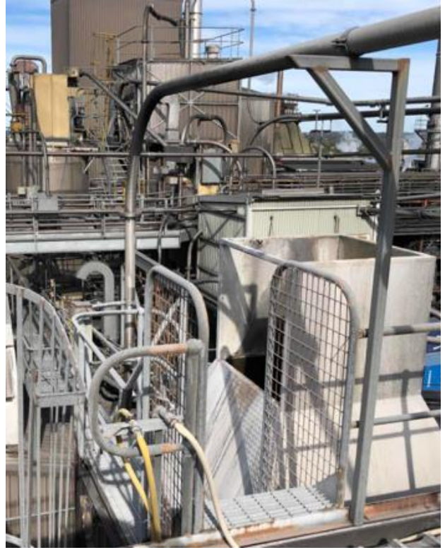
EPA ID 14 – No. 4 Starch Dryer Scrubber
