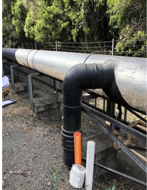
EPA ID 39A - Biofilter Inlet
