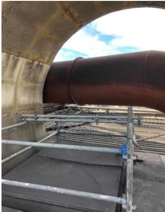
EPA ID 9 – No. 2 Gluten Dryer Baghouse
