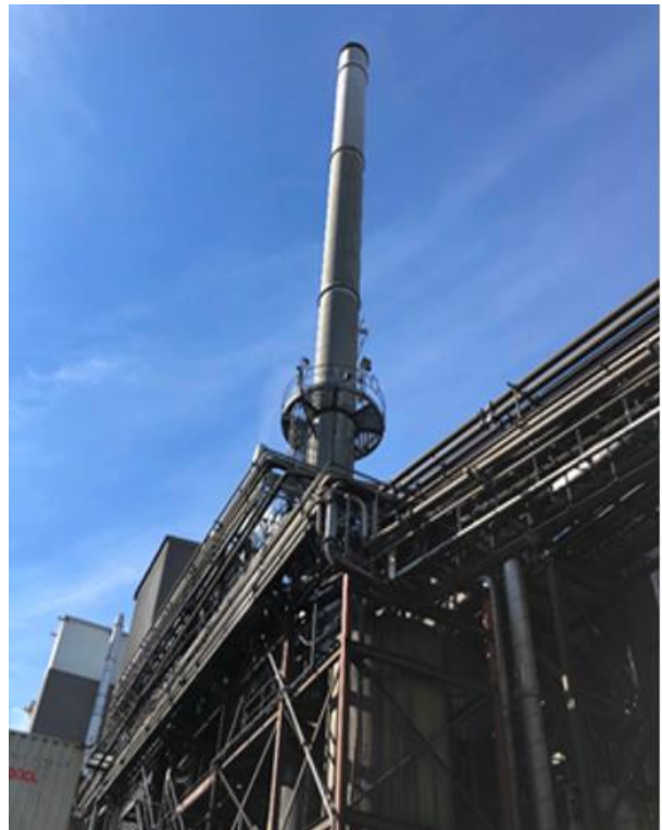
EPA ID 35 - Combined Boilers 5 & 6 Stack
