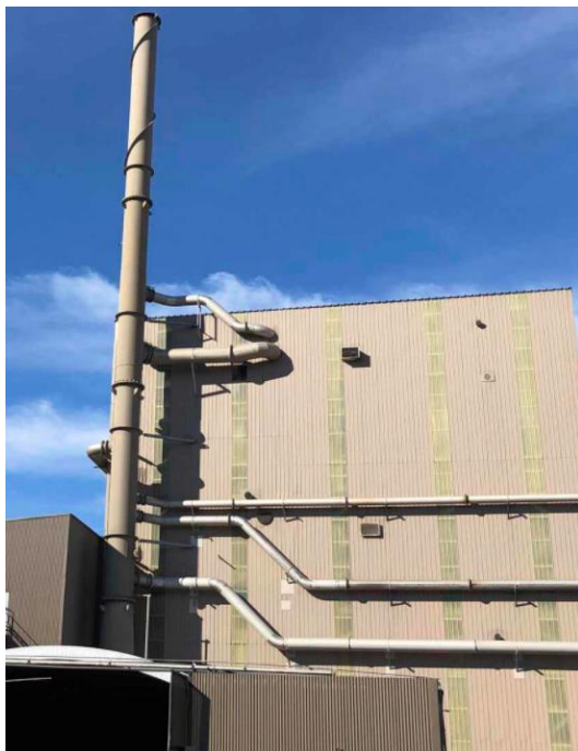
EPA ID 46 – DDG Pellet Plant Stack
