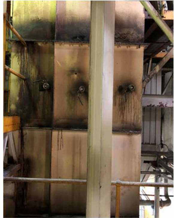
EPA ID 10 – No. 3 Gluten Dryer Baghouse
