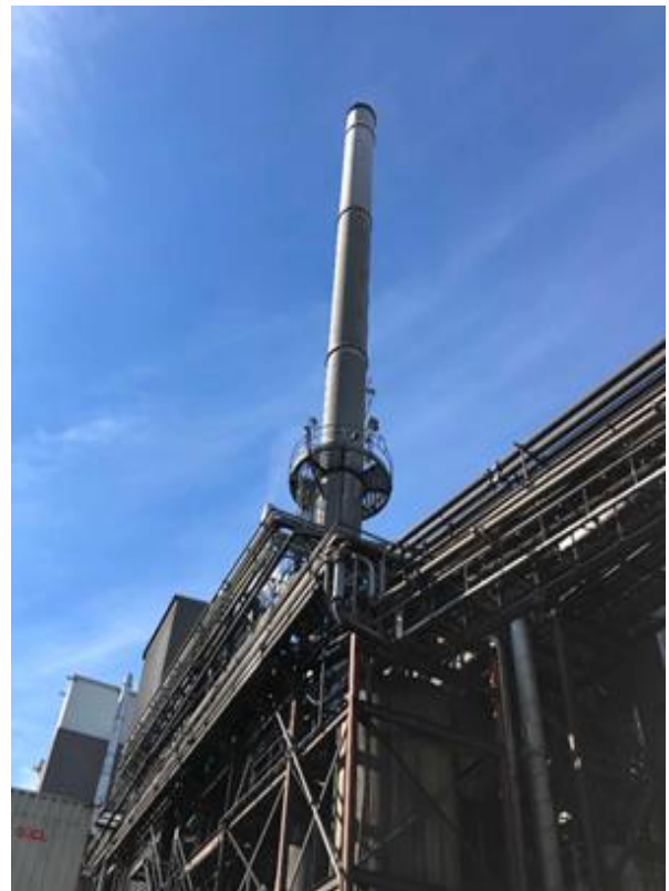
EPA ID 35 - Combined Boilers 5 & 6
