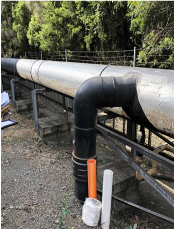
EPA ID 39A - Biofilter Inlet
