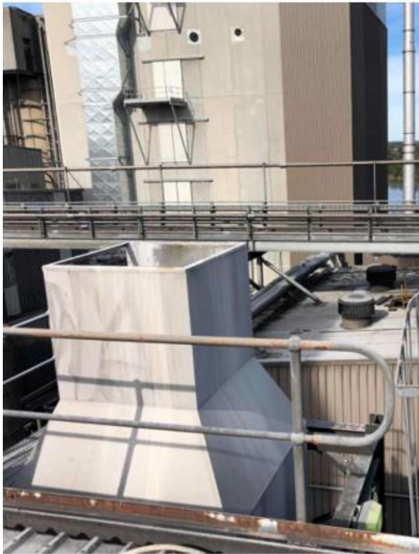
EPA ID 13 – No. 3 Starch Dryer Scrubber
