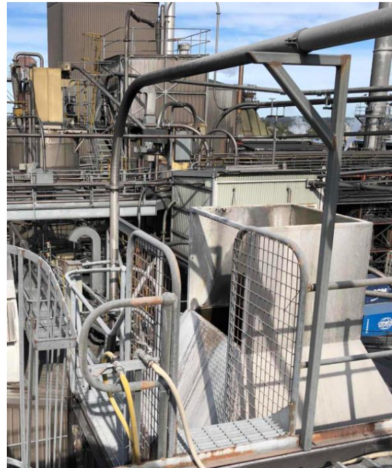
EPA ID 14 – No. 4 Starch Dryer Scrubber
